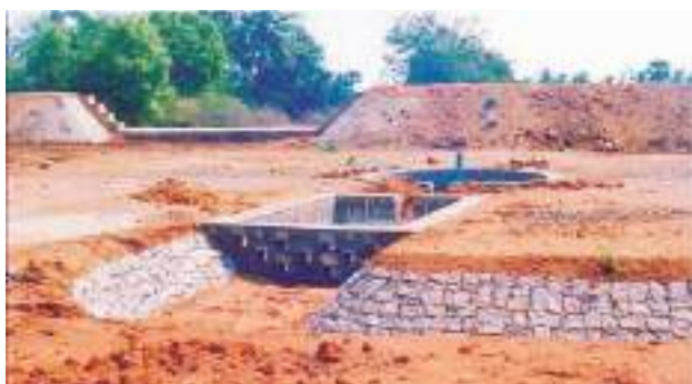
Recharge shaft developed at Coimbatore
